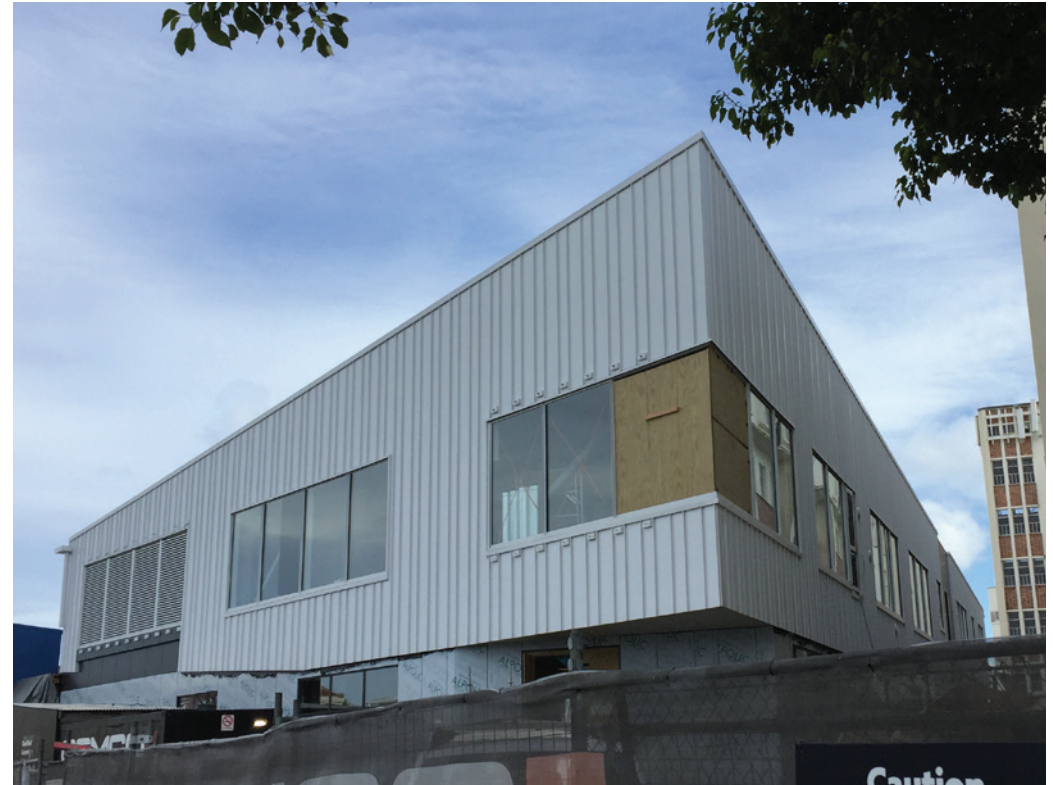
Roofing and cladding supplied by Steel & Tube Roofing on the new Hastings Hospital Endoscopy Unit.
